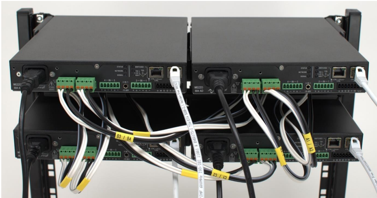
Figure 4.5 - KET setup with 16 channels / 4 Mezzi with KET Mezzo Patch-Bay – back side
