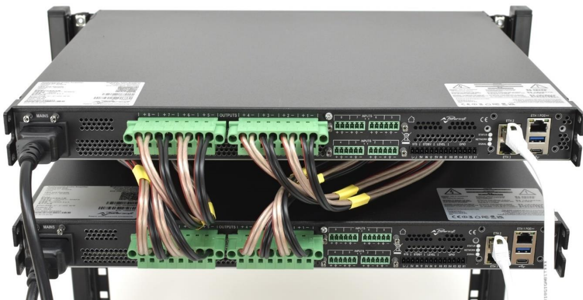
Figure 4.7 - KET setup with 16 channels / 2 Unica with KET Unica Patch-Bay – back side
